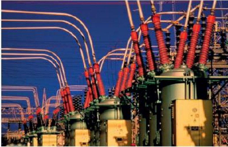
Figure 12.34 Step-up transformers at a power station
