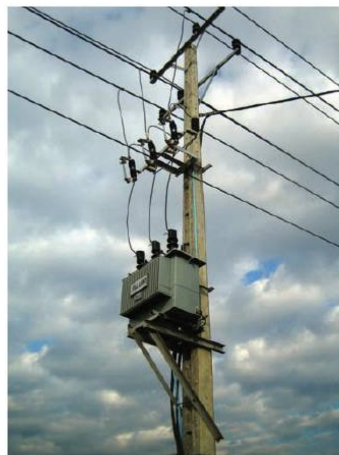
Figure 12.31 A transformer on a road-side pole
