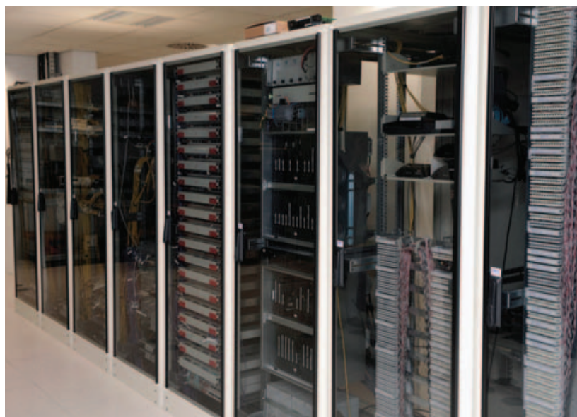
Figure 17.70 A modern automated telephone exchange
