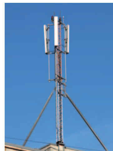
Figure 17.67 A base station with a set of three aerials
