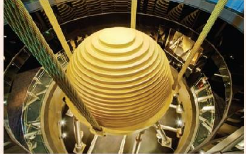
Figure 4.19 The Taipei 101 damper is designed to absorb energy in the event of an earthquake
