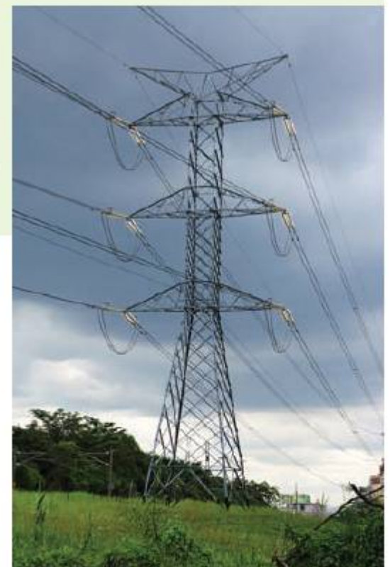
Figure 12.32 Transmission lines transfer electrical power around the country
